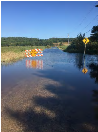
Fish Lake Road Inundated
